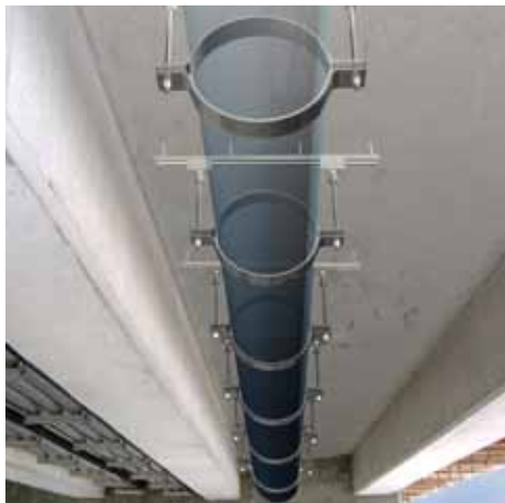
Water Pipelines and other Supports
