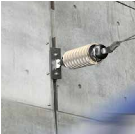
Overhead Electrical Lines
